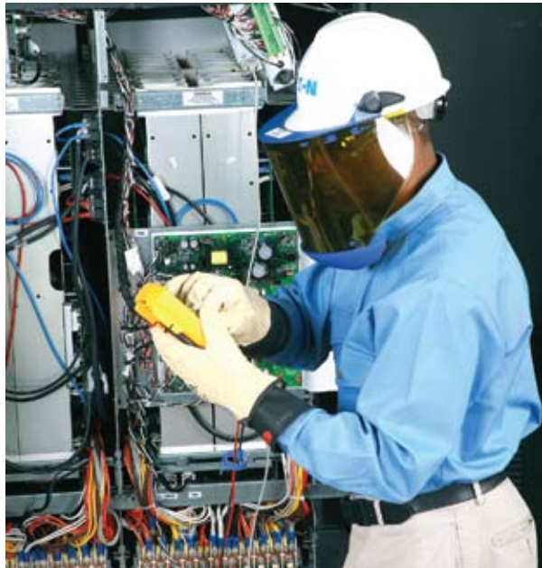
Proper preventive maintenance is critical to keeping systems up and running
