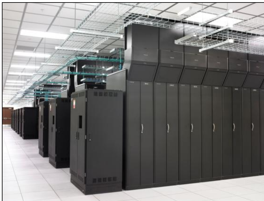
Figure 2: Hot- or cold-aisle containment strategies featuring passive cooling often enable data centers to meet increased density and efficiency requirements more cost-effectively and flexibly than in-row cooling systems.
